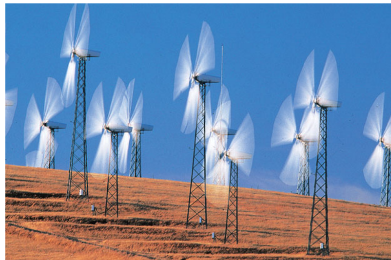
FIGURE 16.15 Windmills on a wind farm near Altamont, California, a mountain pass region east of San Francisco.
