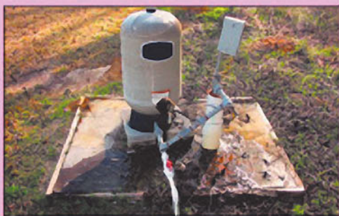
Domestic well, Early County, Georgia
