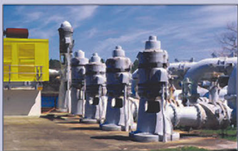
Public supply water intake, Bay County, Florida
